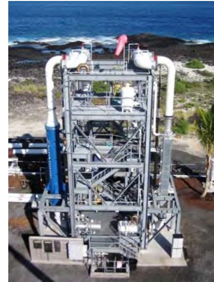
OTEC heat exchanger test facility at NELHA
