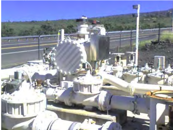
Hawaii County Dept. of Water Supply's 45-kW in-line hydro plant in Kona
