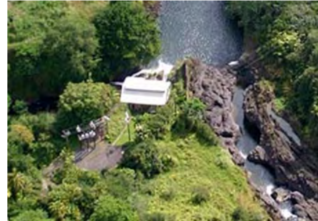
1.1-MW Waiau Hydro Power Plant on the Wailuku River, Hilo
